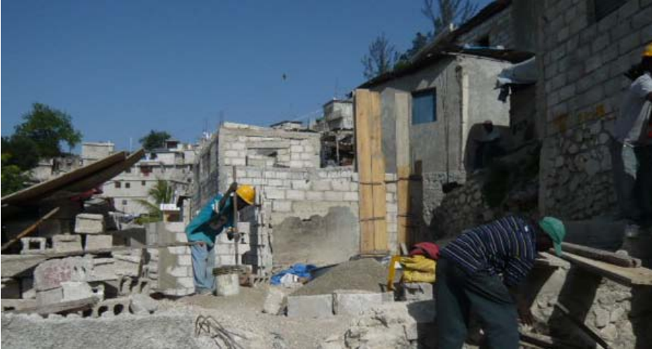
A home repair underway using the training and building guidelines taught by Build Change, June 22, 2011. Photo delegation.
